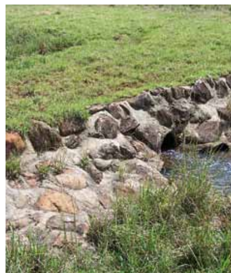
A stock crossing constructed over Arley Creek. This structure will prevent bank damage by livestock thereby minimising erosion and sedimentation of the creek.
