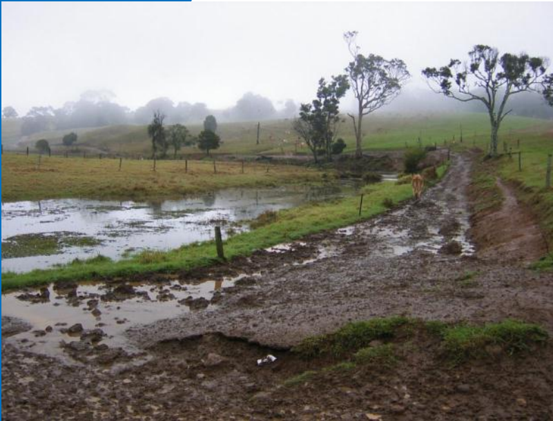
The Hopper property in 2005 following heavy rainfall. Note the proximity of the laneway to Walkers Creek and severe erosion.
